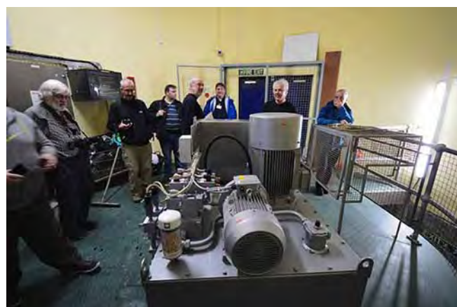
Hydraulic power pack inside the East Quay control room - this pumps oil in and out of the large hydraulic rams which raise and lower the gates. There is one hydraulic power pack per ram and one ram per gate. The hydraulic packs have back-up oil pumps which can be switched over in the event of mechanical failure
